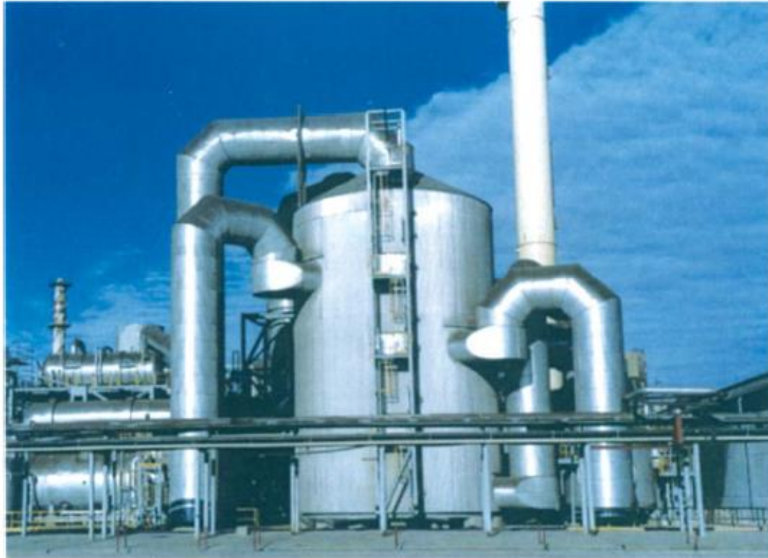
Fig. 7.7. Photograph of catalyst bed converter, courtesy Outokumpu OYJ www.outokumpu.com . Gas inlet and outlet flues are shown. Others are hidden behind. Fig. 7.6's gas coolers are also hidden behind. Converter walls and roofs are designed to be strong enough to withstand their acid plant's main blower 'shutoff' pressure without damage (Friedman and Friedman, 2004). Catalyst 'tray' supports are also strong enough to withstand the downward force exerted by the descending feed gas (at the converter's operating temperature).
